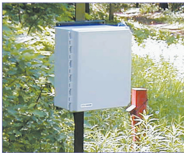
Remote Telemetry Station
